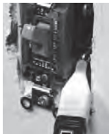
AC Voltage in switches
