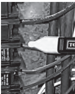
AC Voltage in junction boxes
